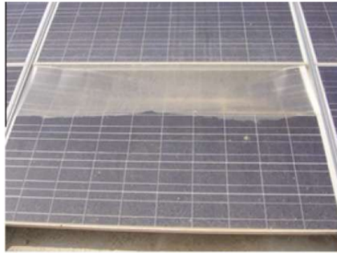
FIGURE 2. A PV module with delamination [10]
